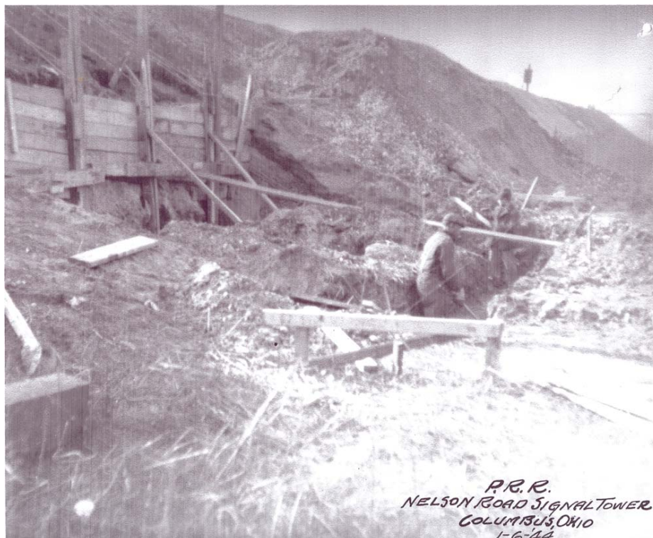
Figure 1 – January 6, 1944 work starts on the foundation. AC Tower was located just west of Nelson Road on the north side of the tracks. The camera is looking west. In 2020 the tower is gone. The site still shows up on Google Maps.
