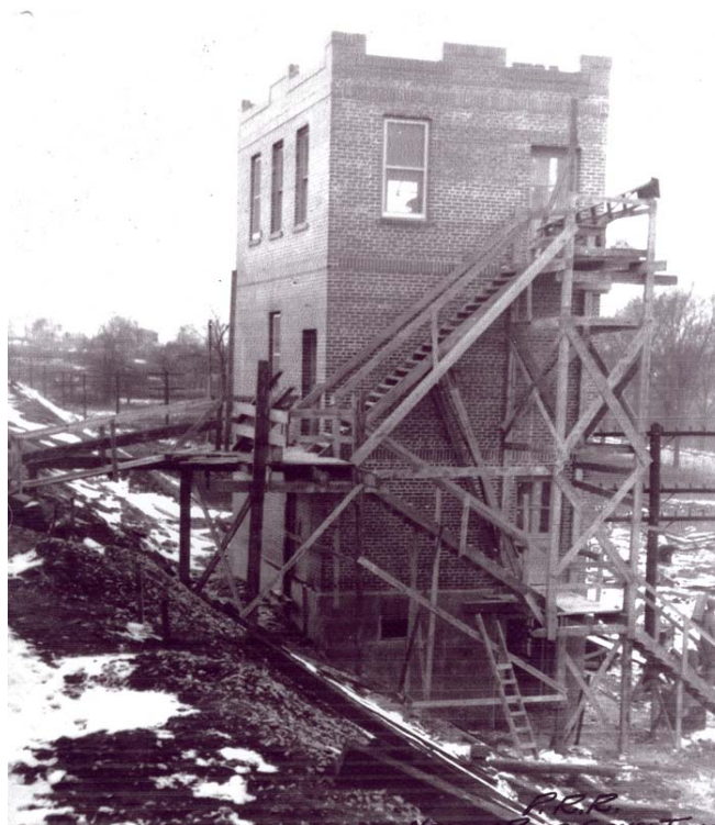
Figure 5 – March 1 the brick work is nearing completion. Windows and doors have been installed.
