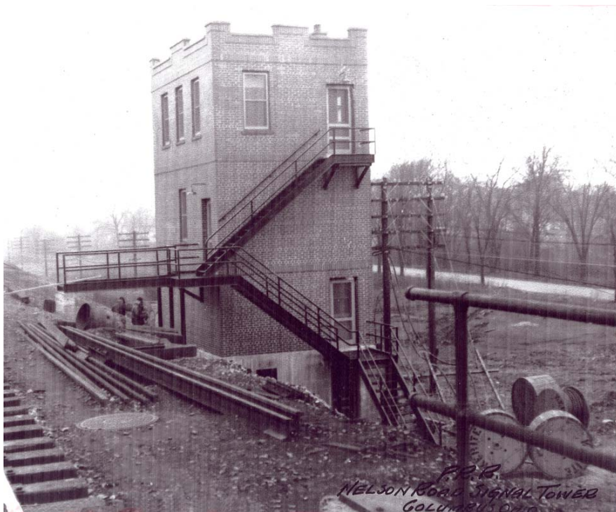
Figure 7 – AC Tower is complete with equipment to control the switches and signals being installed and wired.
